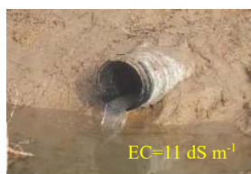
High-salinity leach water is discharging into an open ditch.
