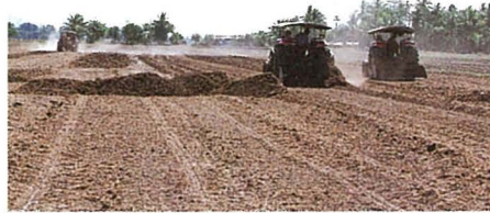
Land levelling using a tractor with a rear bucket. (Photo by H. Fujii)
