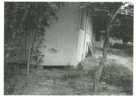
Photo: Damage of structures built on collapsible soil
