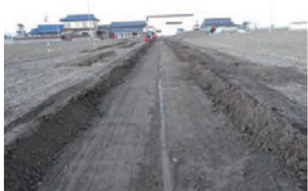
Fig. 11. Treated surface and rows of discarded soil after reciprocating removal work using modified type of embankment topsoil removal machine
