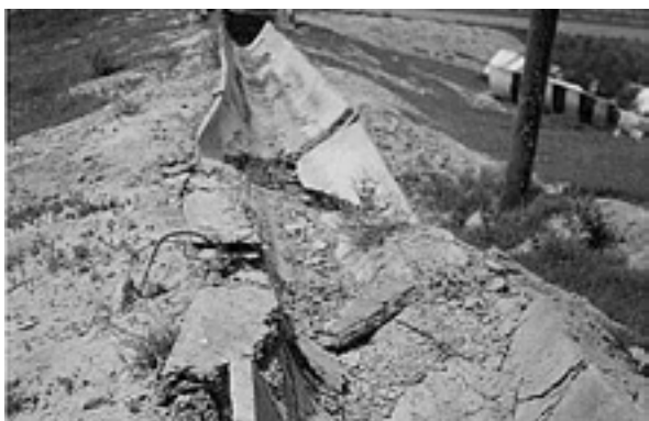
Fig. 2. Deteriorated irrigation canal
