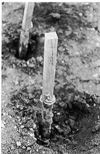
Plate 3. Appearance of damage
