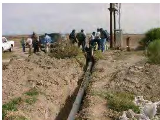
Embedded pipelines of the water supply system as part of water conservation efforts to prevent evaporation and improve irrigation efficiency
