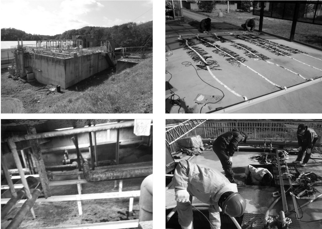
Fig.2 The wastewater purification facility for swine waste surveyed in this study.
